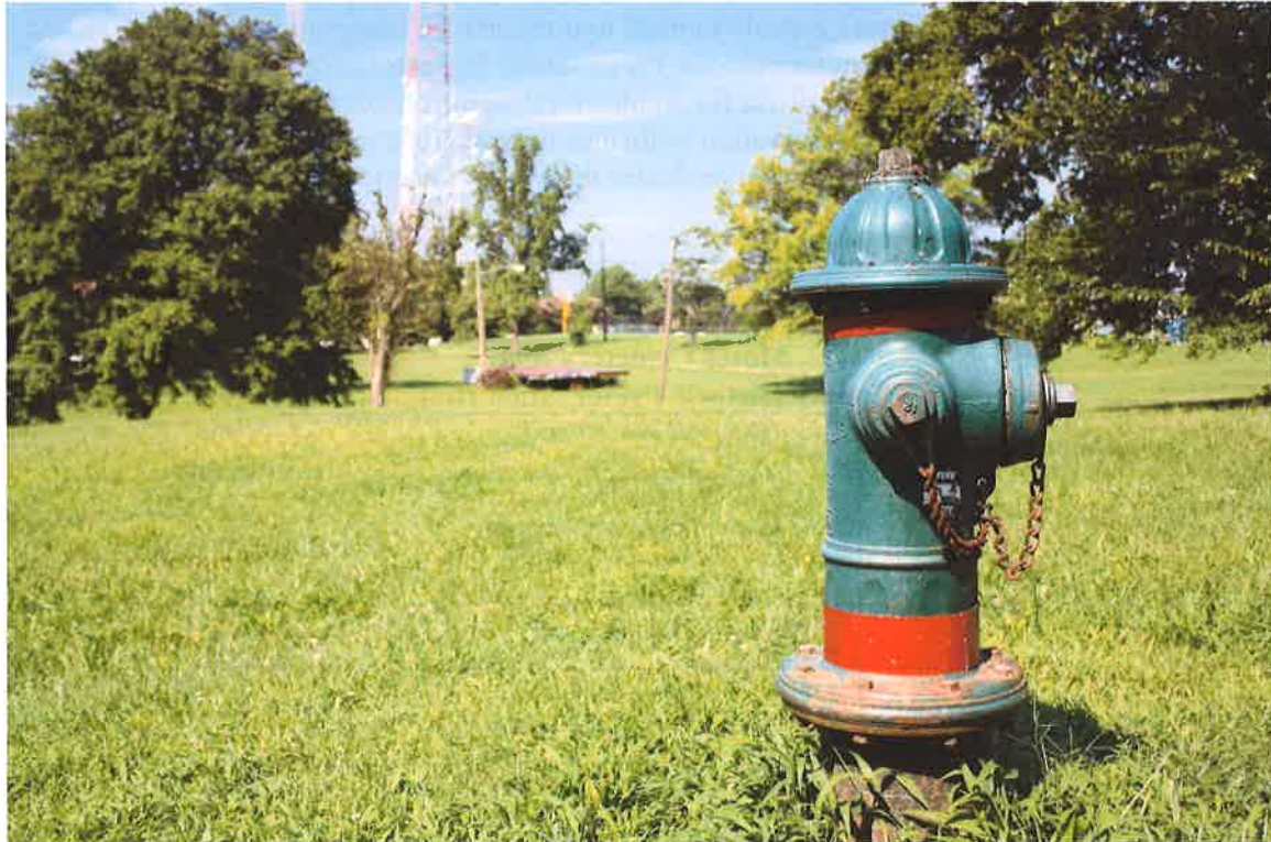
Figure 31. Fort Reno Park, fire hydrant in the vicinity of the former 3812 Davenport Street.
